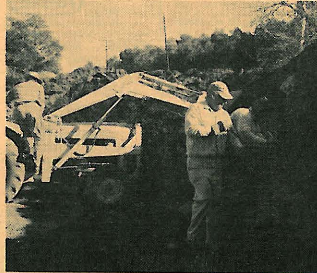
PICTURED ABOVE IS JIM SOCKWELL, JACK HOISTAD AND TOM JUDD AS THEY ARE WORKING ON REMOVING A CULVERT IN PREPARATION FOR CLEARING THE LOT BELONGING TO JERRY FUNK.
